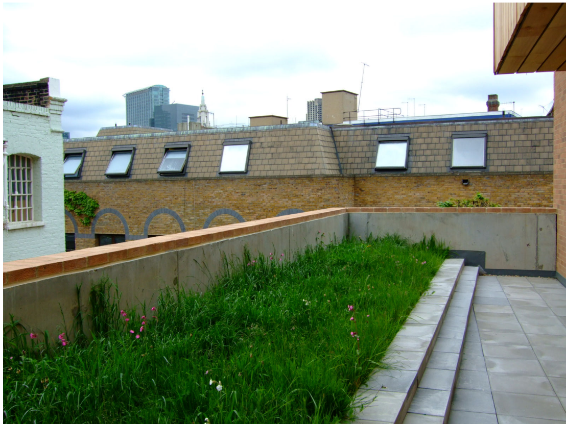
Smaller of the two roof terraces, at the south-west corner of the building
